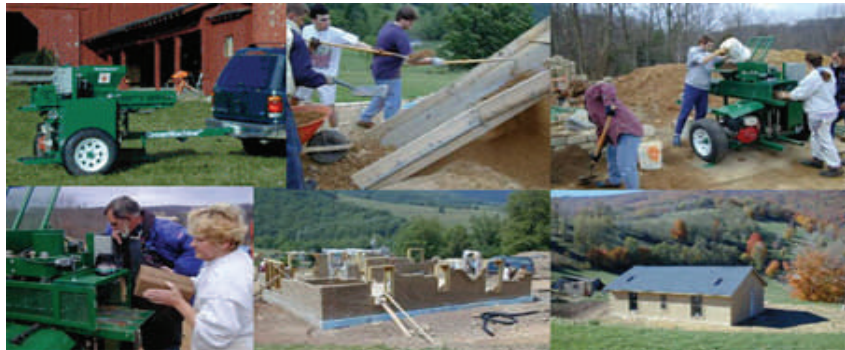
The stages of construction of an Earth Home designed by John Spears
