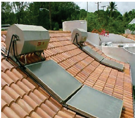
Rooftop solar hot water heater
